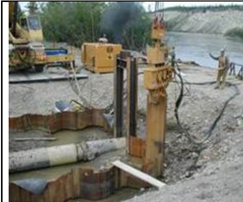
Photo 1: Install the sheet piling using a vibratory hammer hoisted by a crane.
